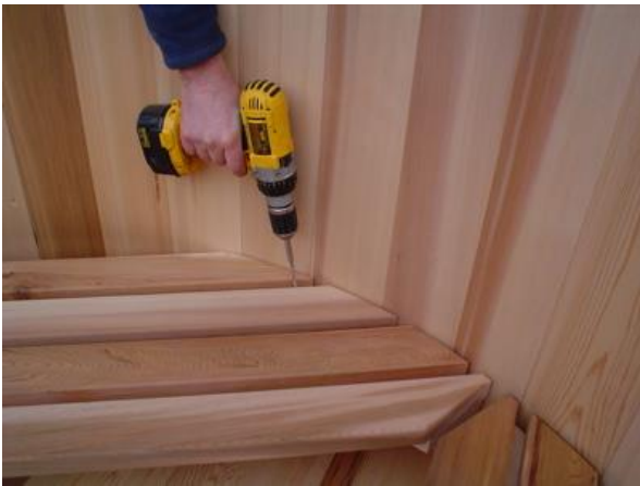
Figure 9.3 Attach benches to bench blocks with 3" stainless screws between the bench slats into the tops of the bench blocks
