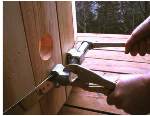
Figure 8.2 Using pliers to resist as you tighten. Stop when you see noticeable deflection of the aluminum blocks. This indicates bottom strap is tight enough. Upper straps should not be as tight.
